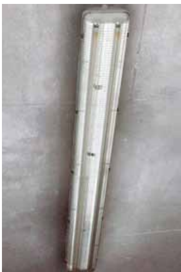
Artificial lighting with unbreakable cover
