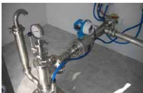
Inside view of the head of a borehole designed to avoid contamination and to allow sampling
