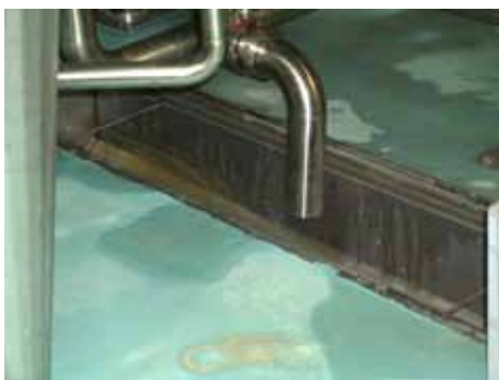
High capacity drain in a bottling area
